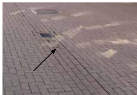
Channel - Buff concrete paviours (running)
